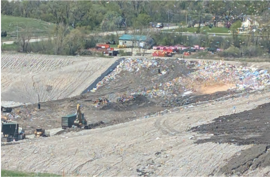
North end of Phase 4, needs additional cover
