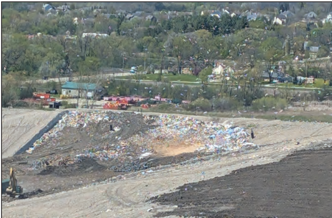
North end of Phase 4, needs additional cover
